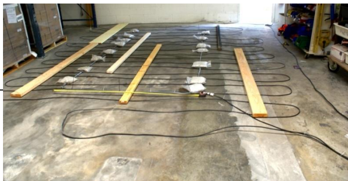
First snow melt system laid out, the cable was so thick that we used wood boards to help press it down over a weekend before running the test.
